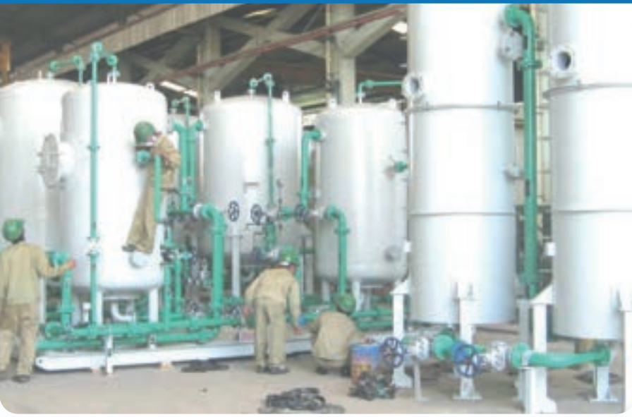
Flash Mixing & Flocculation Tank
