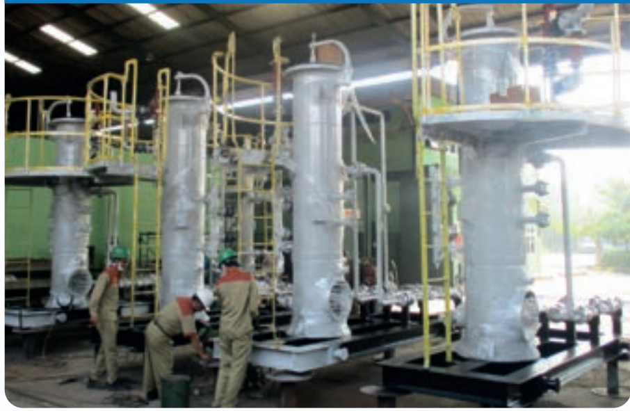
FUEL SURGE DRUM
