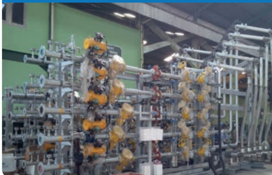
Structural & Skid Metering
