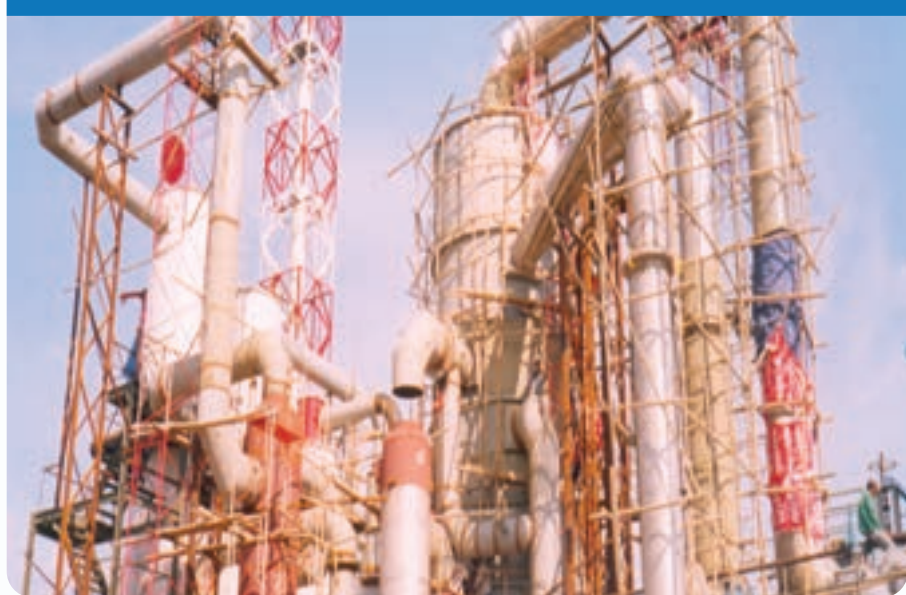
SULPHURIC ACID PLANT
